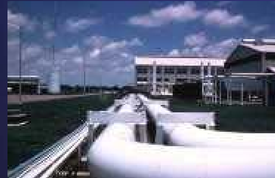
Valve and Pump Control
