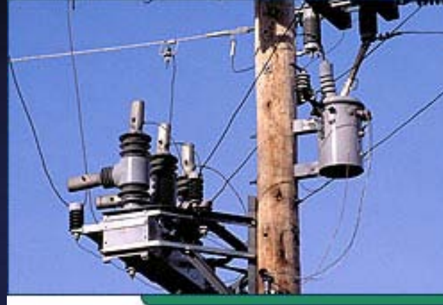
Voltage Regulators, Capacitor Banks
