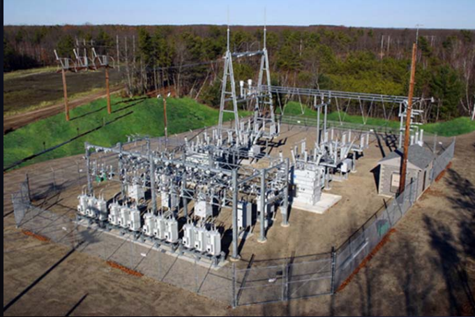
Transmission & Distribution Substations
